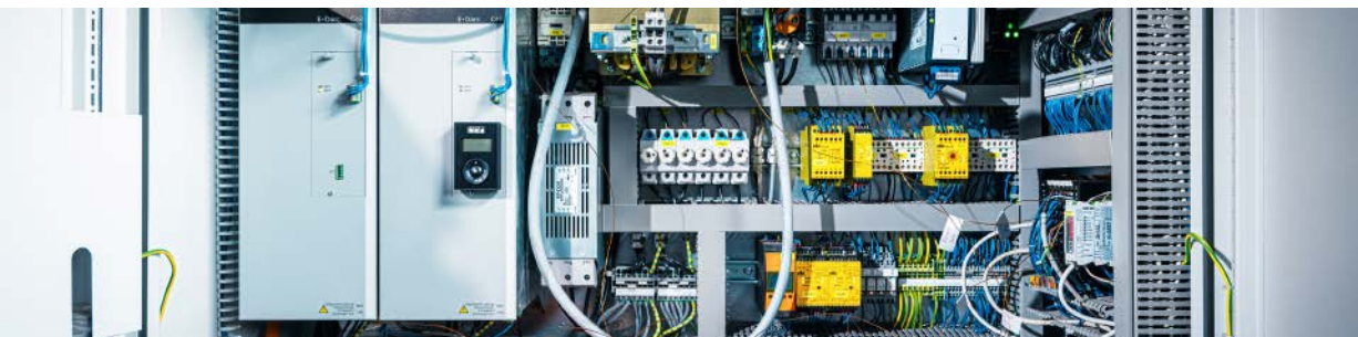
➤ Goal achieved: sustainable reduction of energy consumption through DC link coupling. A look inside the control cabinet reveals the E°Darc 48 high-speed servo controllers. The company subsidiary Eckelmann FCS used them to implement the drive technology for the test stand, which has a maximum output of 52 kW but only consumes 2 kW from the mains.
